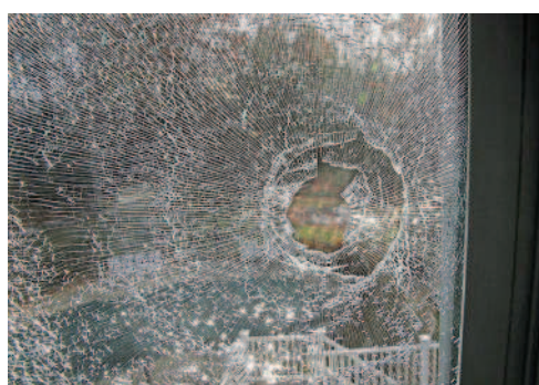
A second story bathroom window was punctured by a bullet coming from the woods behind 86 Hidden Valley Drive in Dover.
